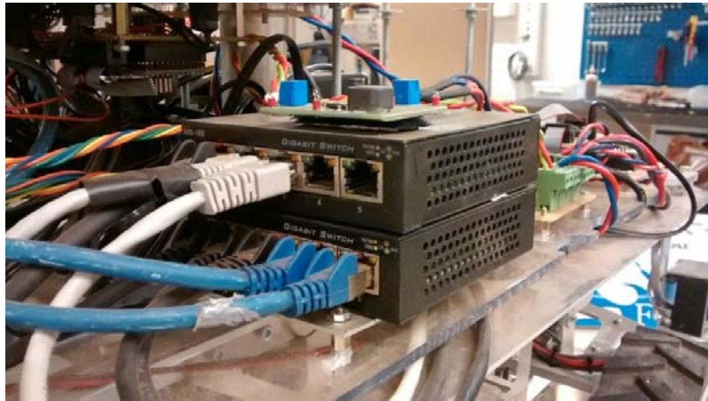
Figure 3.26: Twin D-Link DGS-105 Ethernet Switches
